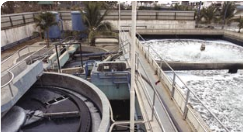
Photo: Proper wastewater management requires that effluent go through various stages of treatment before it is discharged.
